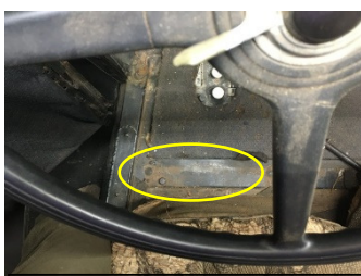
Looking straight down from the driver's seat, showing where on the body cross member to look.
