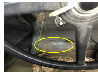
Looking straight down from the driver's seat, showing where on the body cross member to look.
